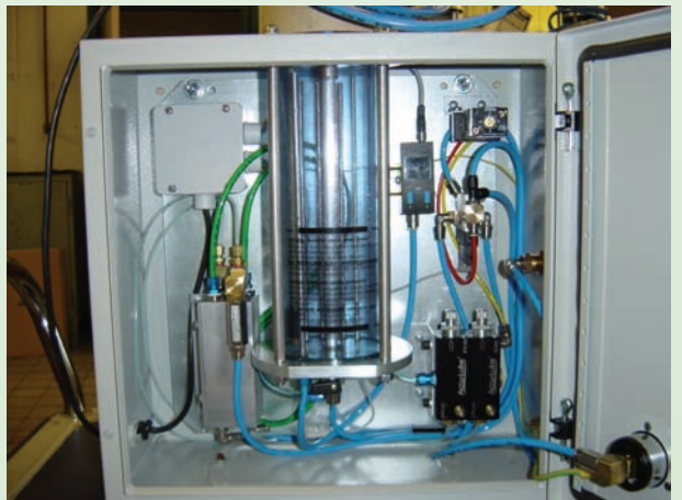
2 pumps for inside lubrication
