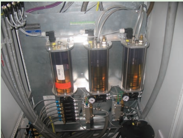
6 pumps for outside lubrication 4 pumps for inside lubrication
